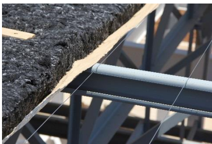
Fiber Over Purlin Suspended on Wires Airport
