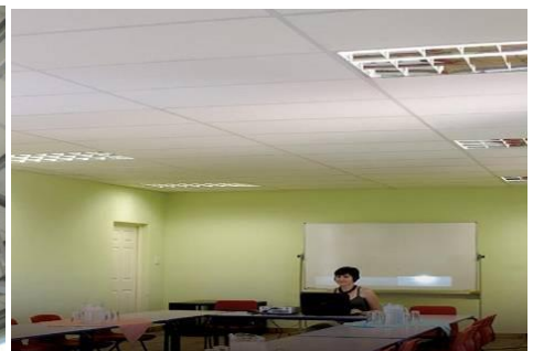
Suspended Ceiling Vinyl Faced Board 600mm x 1200mm Board Room
